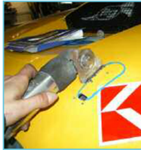
After marking AeroCatch and stud strike positioning, cut out shape from panel.
